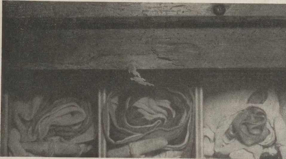
Shown above is the flag locker on the bridge of the lake tanker Boscan , illustrating ravages of termites.
